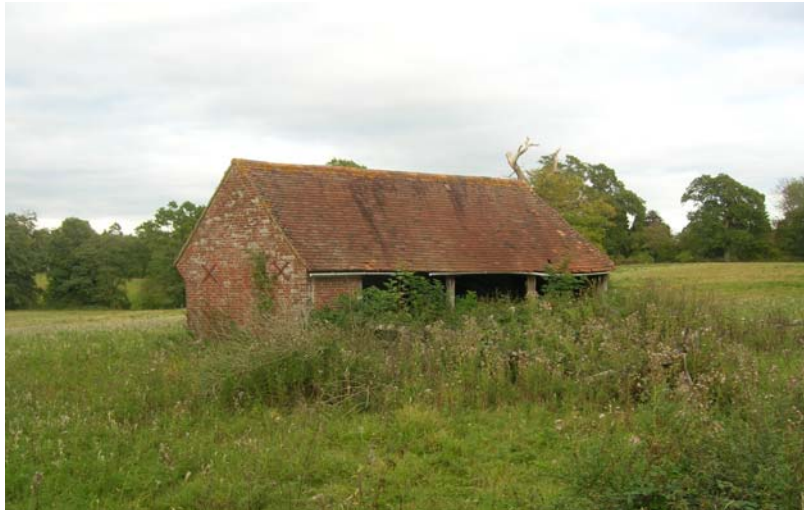
Poor condition of barn along Church Lane
